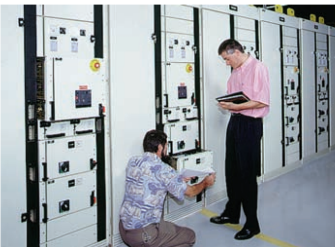
Motor Control Centre (MCC).
